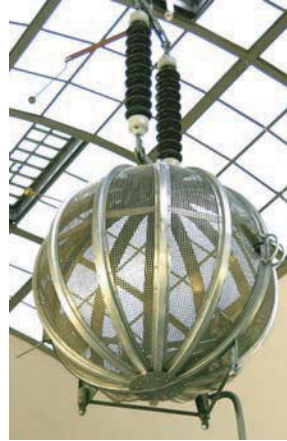
Faraday cage: to capture / shield energy pulses
